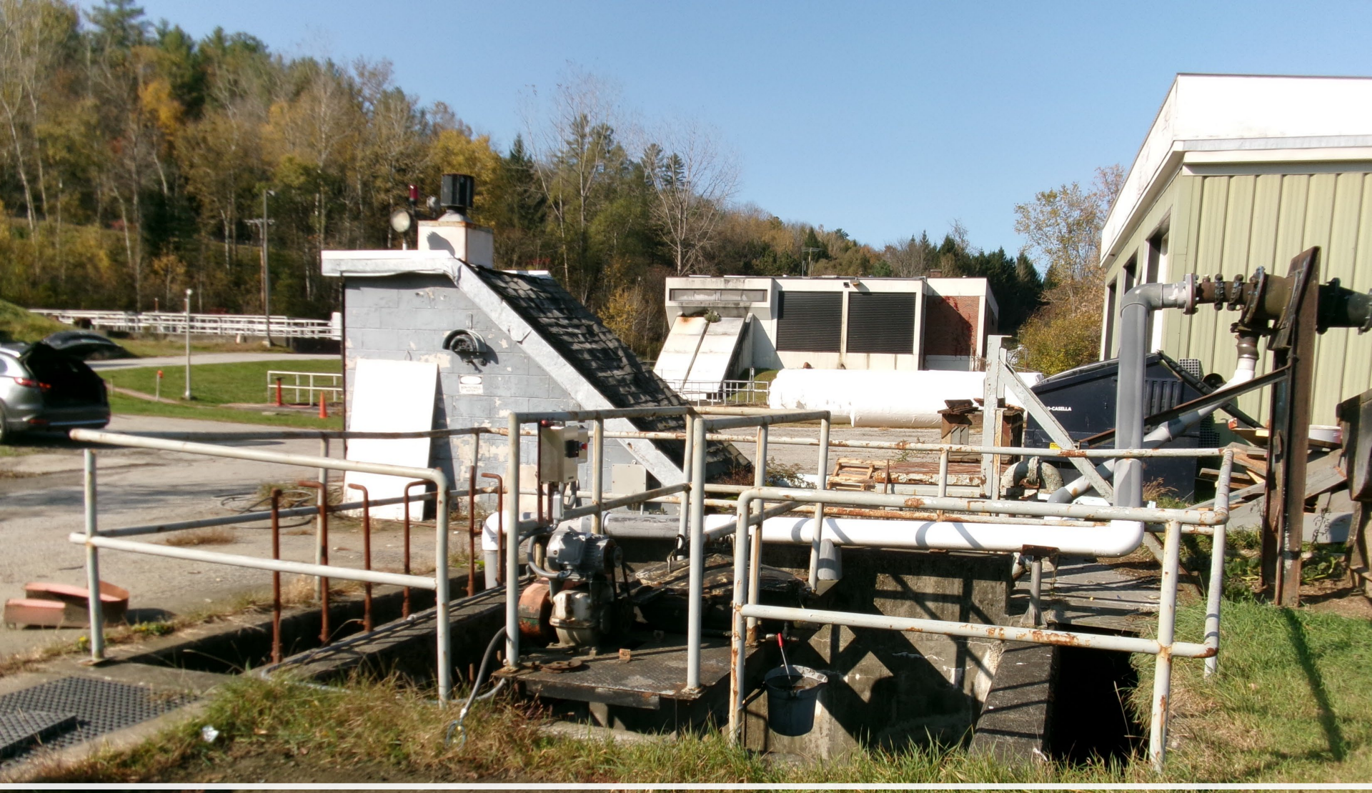
Existing Grit Removal System
