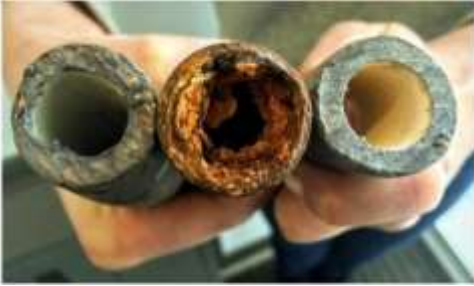
Lead service pipes. Photo courtesy of the Environmental Protection Agency via the Vermont Department of Environmental Conservation
